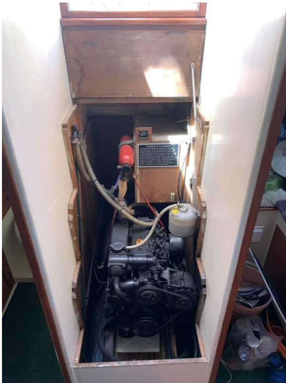
Main engine under stairs, looking aft, centerline
